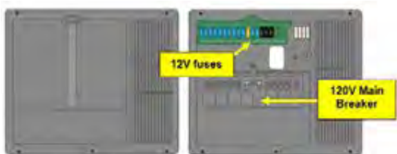
Typical Load Center Panel
