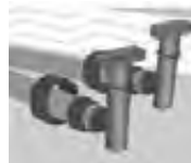
Low Point Drains
