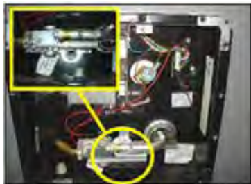
Fig 1: Water heater drain plug
